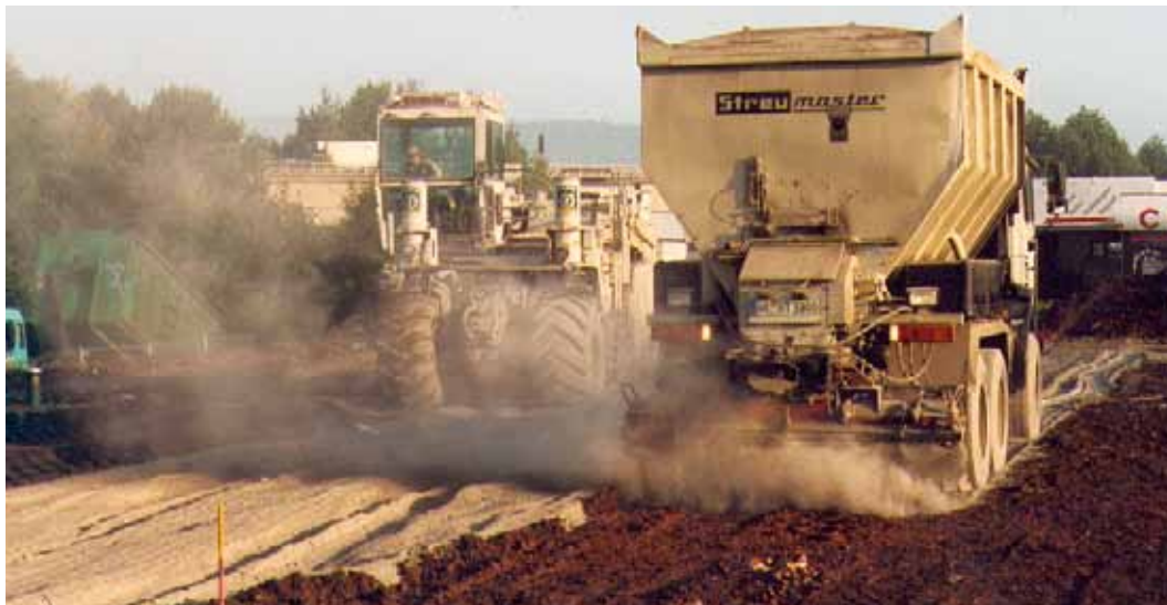
Fig. 2: The special binder NovoCrete® is applied over the base course with a binder sprayer and milled 0.30 m deep into the in-situ earth with a Wirtgen® WR 2500.
